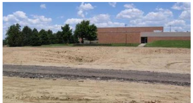
Leveling the land to be used for the new Anita Recreation Center is the first step in moving from a dream to reality. The Center will be located in close proximity to the Anita High School (pictured in the back).
